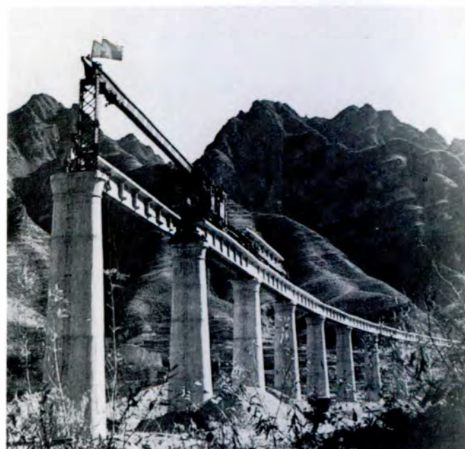
The photo shows a reinforced concrete beam being emplaced on completed piers. Opening up rail lines through this rugged and remote area is a striking example of the central government's determination to develop the Southwest and to firmly integrate it with the rest of the country.
